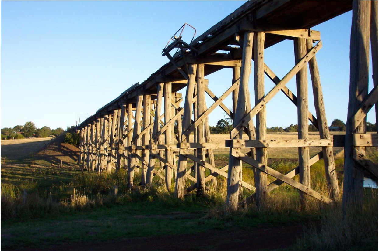
Historic Trestle Railway Bridge over the Grange Burn waterway, Young St-Elizah St, Hamilton (Photo: B. Warton)
